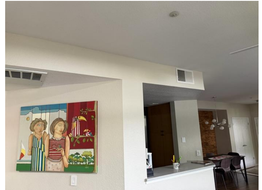
Air handler & heating vent
