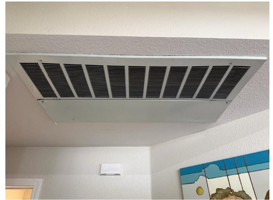
Air handler intake with a filter
