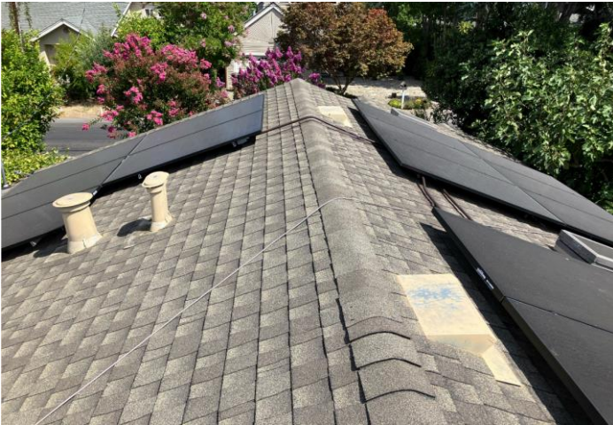
Figure 9: The solar array on all planes of the roof to maximize solar production to offset utility bill costs.
