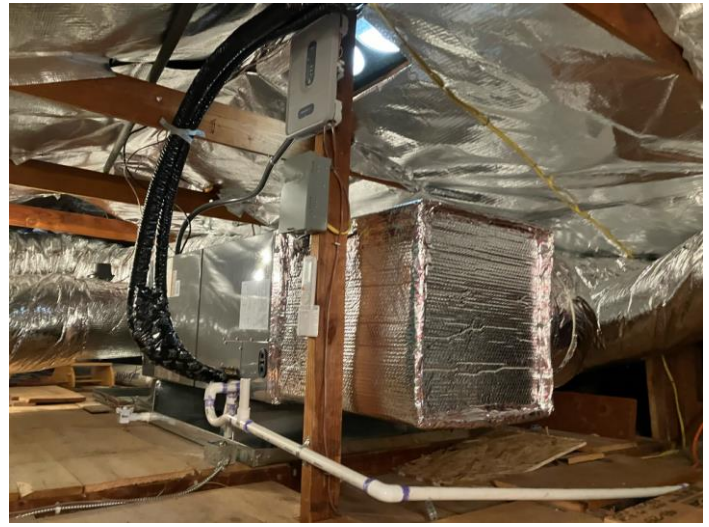
Figure 8: The new HVAC system installed in the attic, with ample insulation around the heat pump itself, and on the lining of the rafters.
