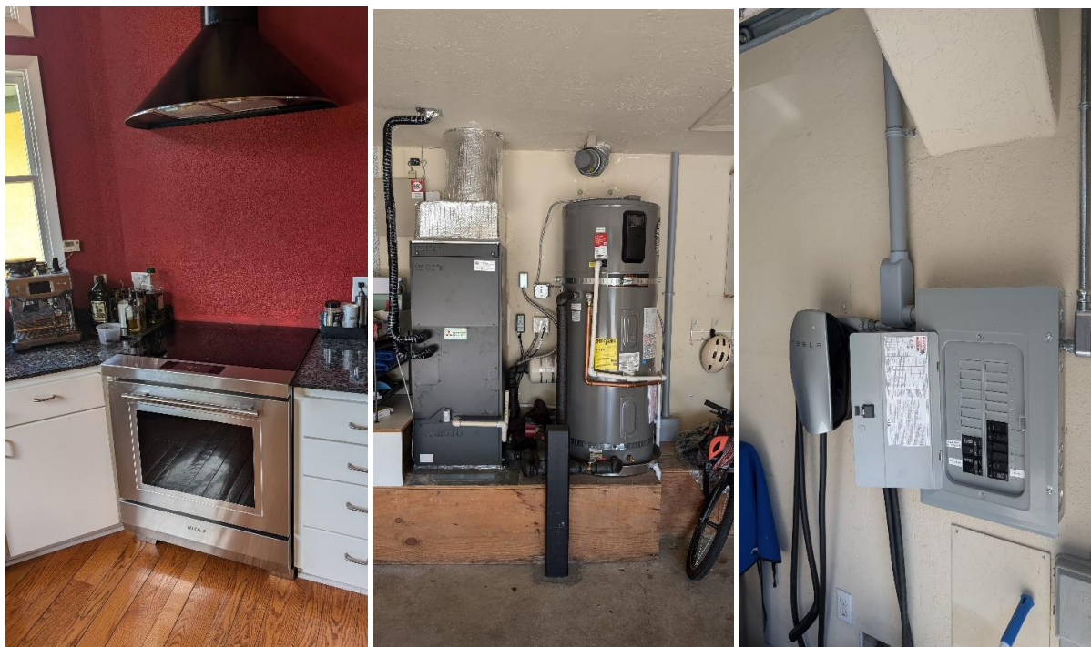
Figure 11: The new electric induction stove, the heat pump air handler and heat pump water heater, and the electric car charger next to the subpanel for the water heater.
