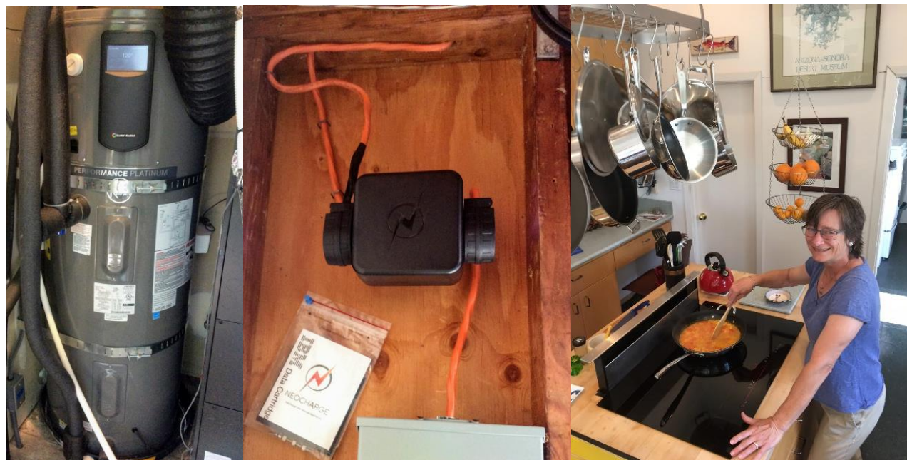
Figure 15: At the Schmidt’s home, the Bosch electric induction stovetop is shared on the same circuit as the Rheem heat pump water heater using the NeoCharge (middle) (Images courtesy of Steve and Lisa Schmidt).
