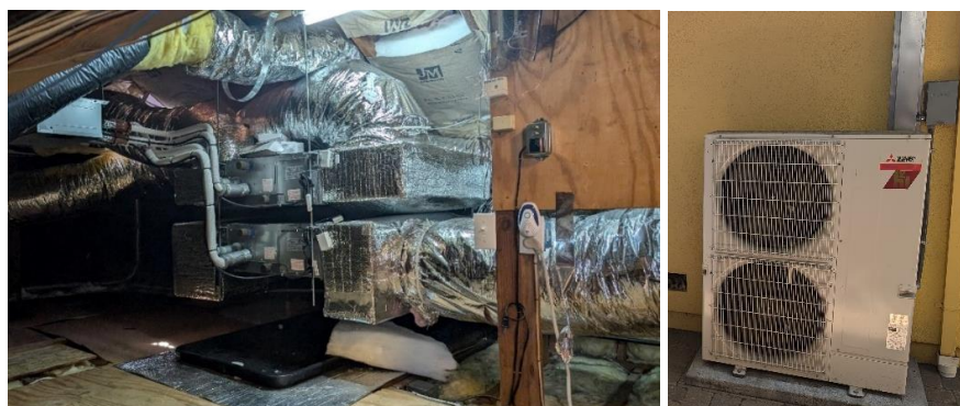
Figure 12: The heat pump air handler in the attic, and the heat pump compressor sitting on the outside of the house.
